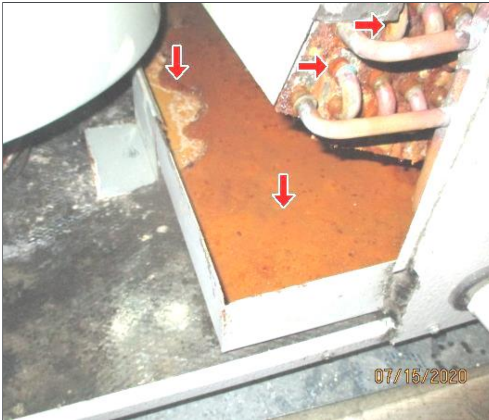
7.0 Item 1(Picture) Drain Pan
